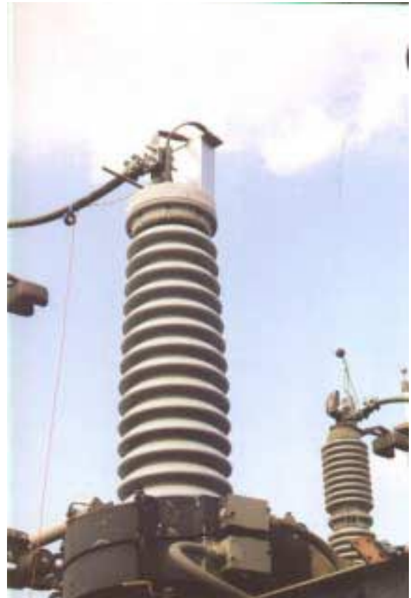
Figure 3: Current shunt and fiber optic link.
